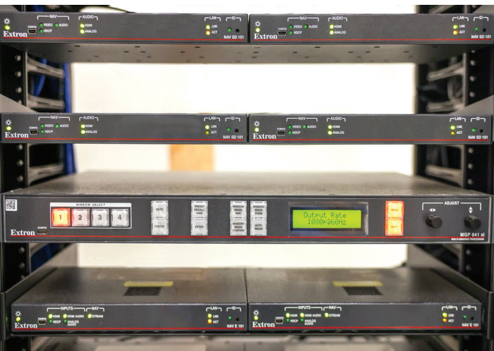
NAV encoders, scaling decoders, MGP 641s, network switches, and other AV equipment housed in racks located in the equipment room.
