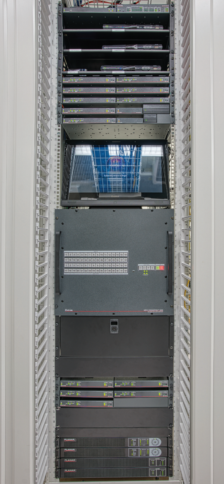
An Extron NAV AVoIP system links the rack-mounted XTP II CrossPoint matrix switcher and the XTP point-to-point installation in the conference room over the center's network.
